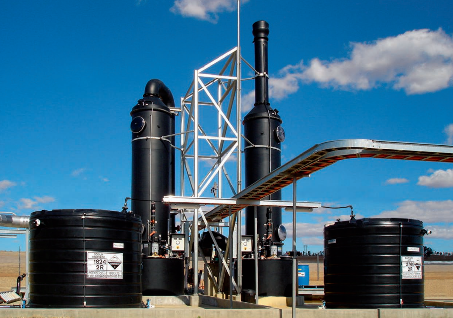
Scrubber plant with fan and chemicals supply tanks located in Australia
