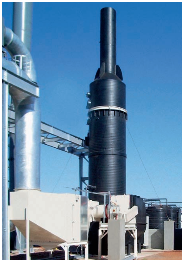
Foundry scrubber for amine KFGV 2000 in South Africa
