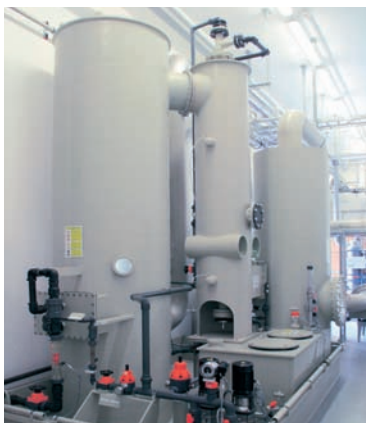
System BAYER-REITHER for \text{SiO}_2 separation in a photovoltaic plant
