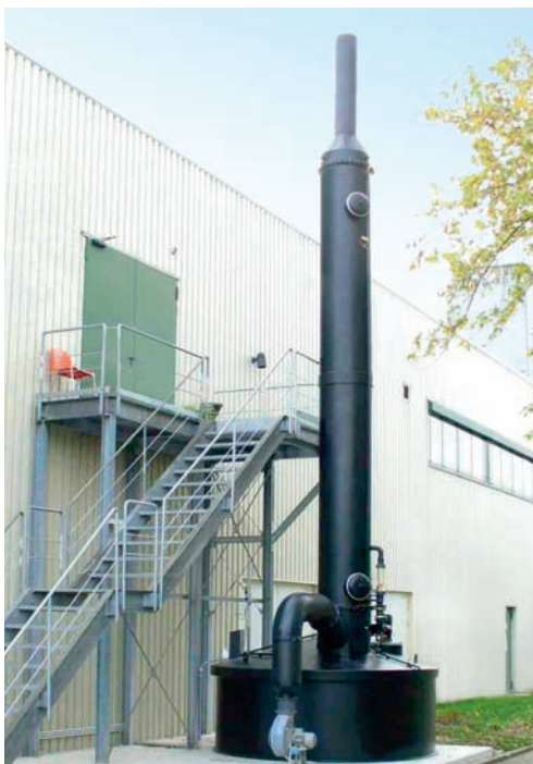
Chlorine emergency scrubber
